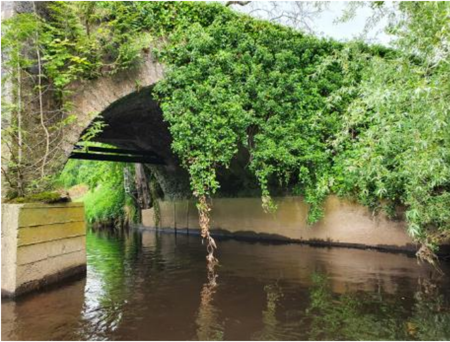
Plate 4-11 - Ivy growing from downstream parapet wall- eastern arch
