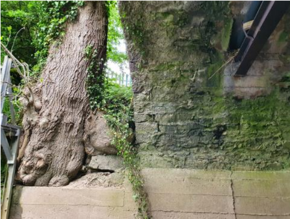
Plate 4-15 - Mature ash with ash die back disease growing very close to bridge wall at upstream western side
