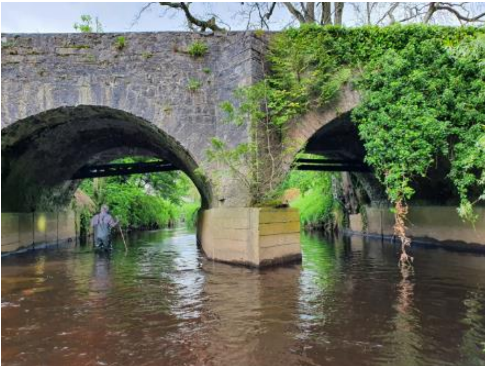
Plate 4-10 - Downstream elevation of bridge showing heavy ivy growth on eastern side of bridge. There is an ash sapling growing on the cement plinth of the breakwater at the downstream face which should be removed.
