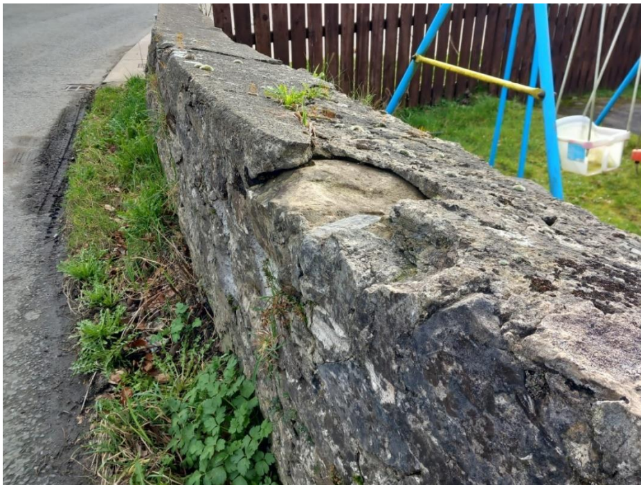
Plate 5: Example of breached capping exposing vulnerable masonry
