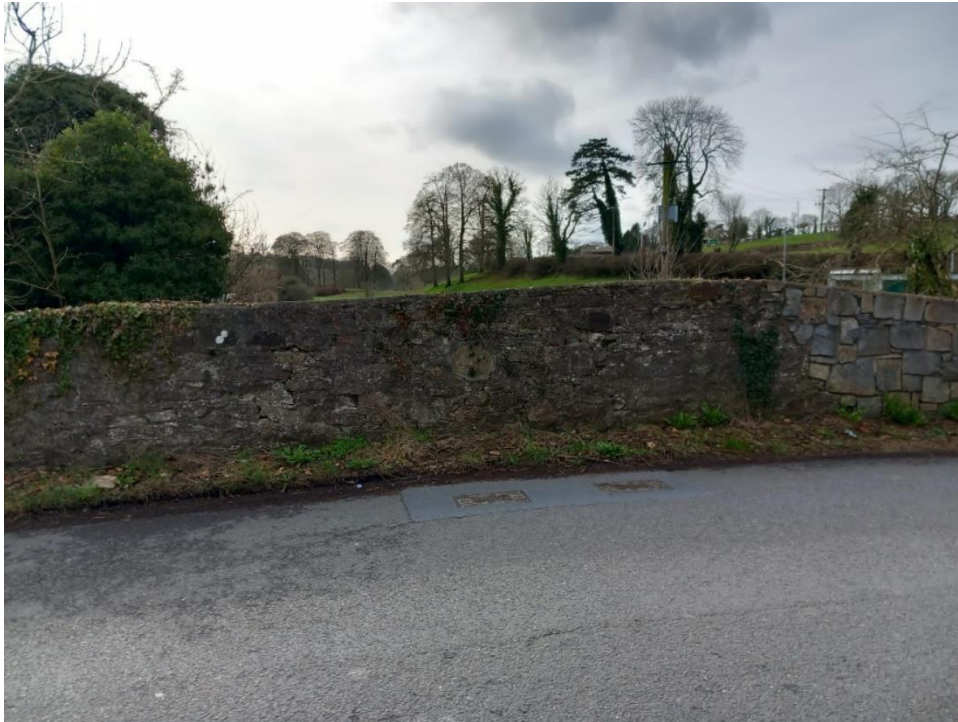
Plate 6: Section of unrepared wall, adjacent to poorly matched masonry infill panel
