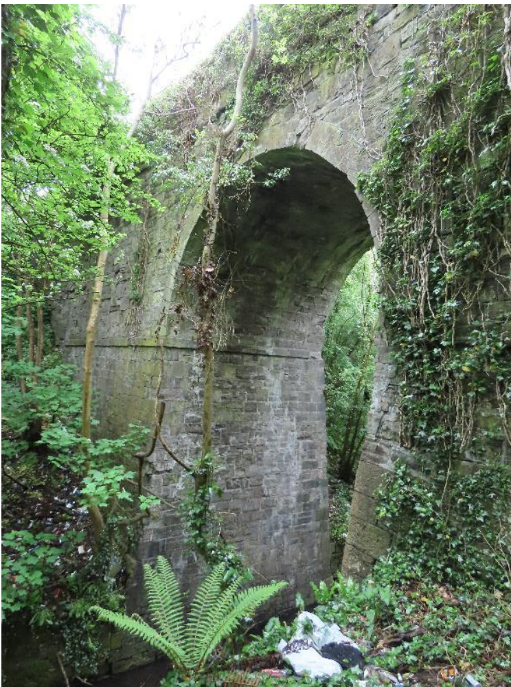
Plate 4-4 - Western elevation of Horseshoe Bridge showing extreme height of structure. This is the side proposed for pedestrian bridge.
