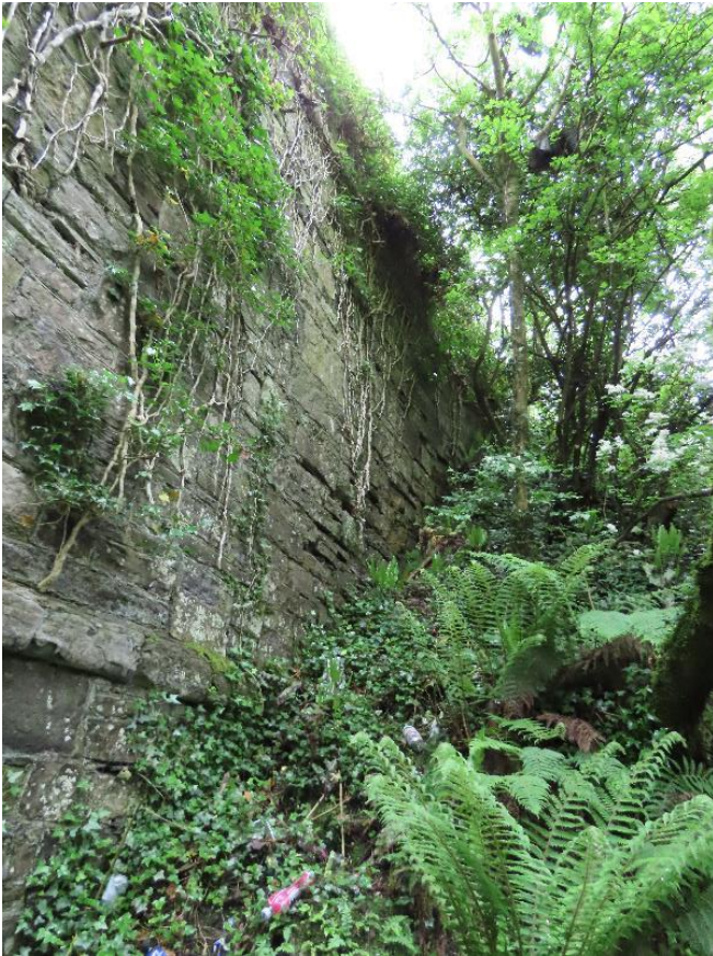
Plate 4-7 - Southern embankment immediately downstream of bridge with immature ash and sycamore with understory of ferns, ivy and brambles
