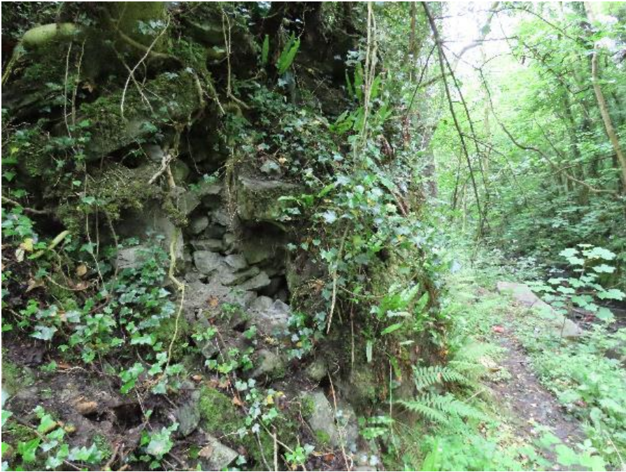
Plate 4-15 - Damage to retaining wall on eastern side of structure on southern bank
