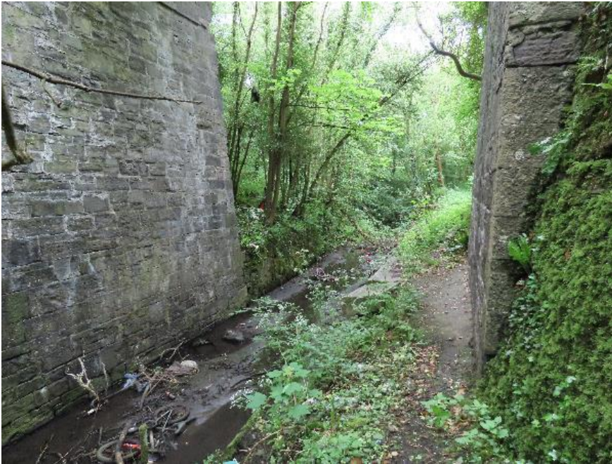
Plate 4-9 - Tow path looking east under structure. Canal channel is dry with a lot of rubbish dumped into it
