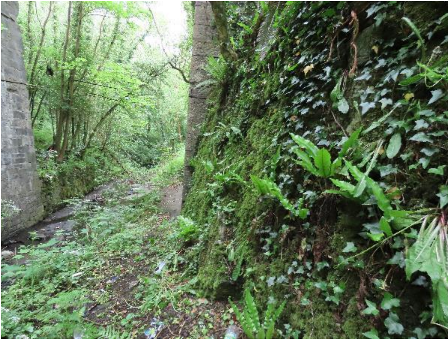
Plate 4-19 - Retaining wall abutting base of bridge on western side on southern embankment
