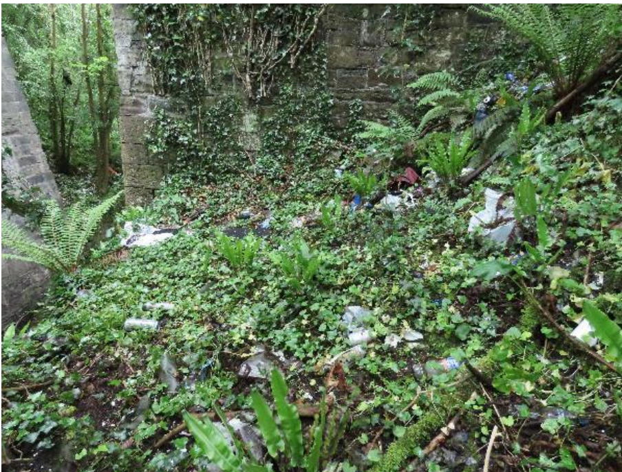
Plate 4-20 - Rubbish dumped from road level lying on embankment
