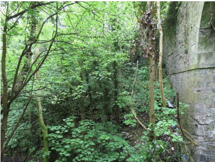
Plate 4-6 - Close up of northern embankment on western side of bridge - vegetation mainly ash saplings and some sycamore
