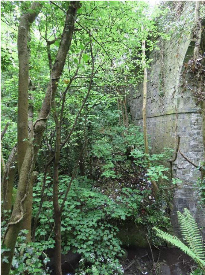
Plate 4-5 - Close up of northern embankment on western side of bridge - vegetation mainly ash saplings and some sycamore
