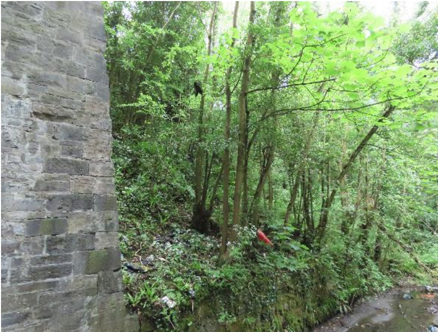
Plate 4-13 - Ash and sycamore saplings growing on eastern side of structure on northern embankment
