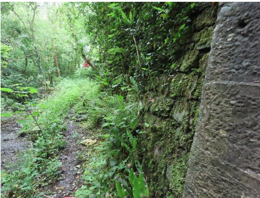
Plate 4-14 - Retaining wall abutting base of abutment at eastern side of structure on southern bank
