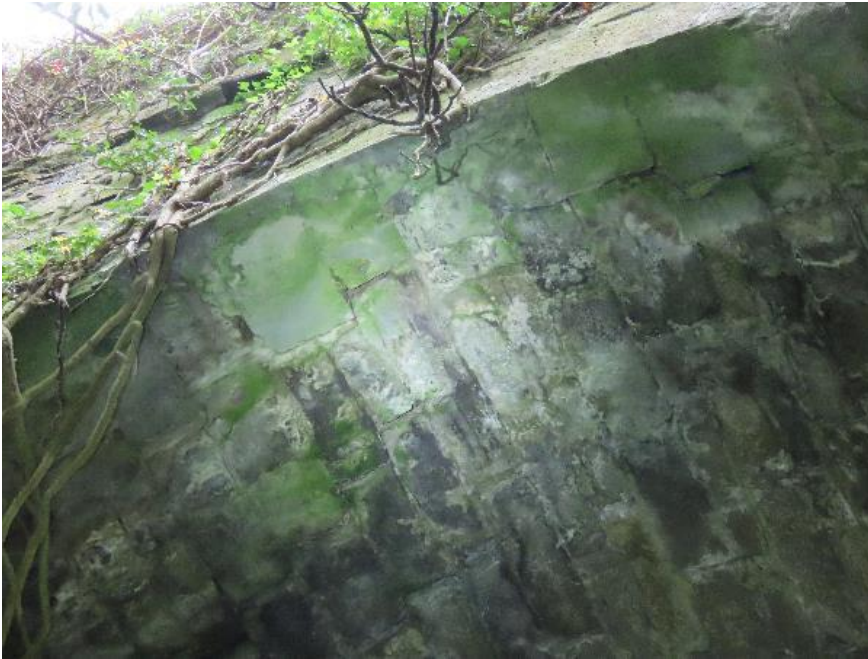
Plate 4-11 - Some suitable crevices for bats under the arch close to the western side of the bridge. It was not possible to mark any crevices due to the extreme height of structure. If under surface of arch is to be repointed this section should be surveyed more closely from a scaffold and crevices selected for retention
