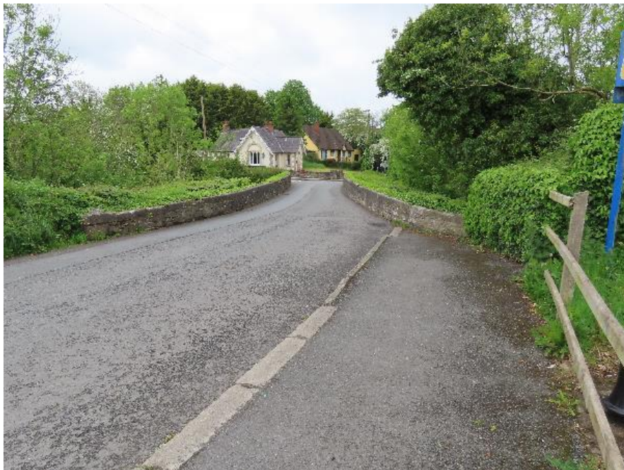
Plate 4-1 - View across bridge looking south showing long parapet walls with ivy growth.
