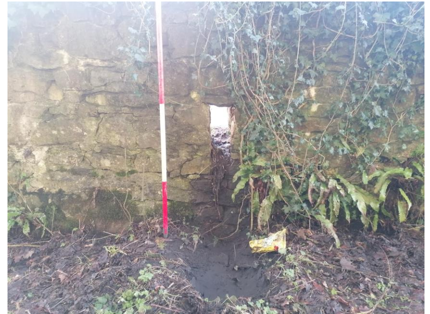
Plate 4: Ballyalbaney Bridge, drainage holes opening onto road
